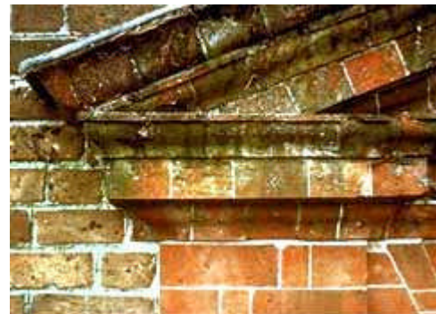
This 18th century pediment and surrounding wall exhibit distinctively different mortar joints. Photo: NPS files.
