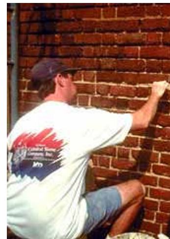
This early 19th century building is being repointed with lime mortar. Photo: Travis McDonald.
